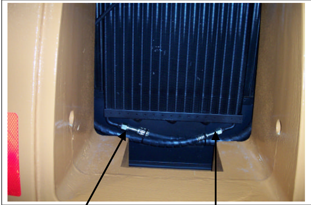
13/32" hose connected to the 13/32" condenser fitting on the left side of the coil.
